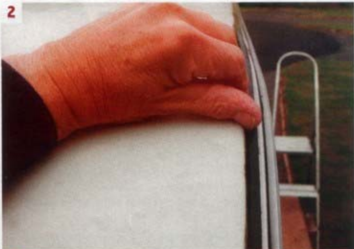
2 ■ On inspection, the awning rail was backed by a rubber base which lacked a suitable sealant
