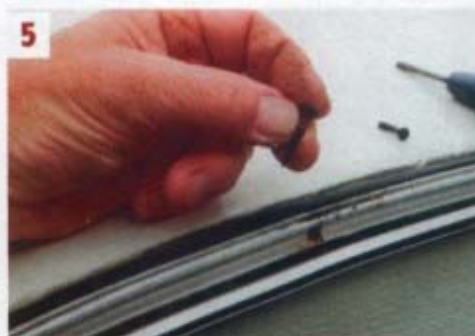
5 ■ A few rusting screws had lost their threads as well – a sure sign that water is starting to creep in where it's not wanted
